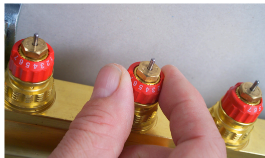
Fig. 8: Preset manifold valve for each heating circuit according to calculations and manifold data sheet.
