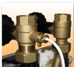
Supply isolating valve with built-in pit for the insertion and the lead sealing of the hot water sensor.
